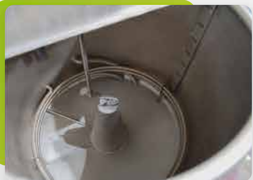
İLAVE KAPLAR İÇİ INSIDE OF ADDITIONAL TANK
