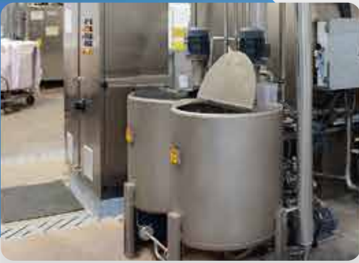
İLAVE TANKLAR ADDITIONAL TANKS
